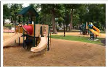
Existing playground was enhanced with addition of subsurface drainage, accessible walkways, safety surfacing and repairs to existing playground
